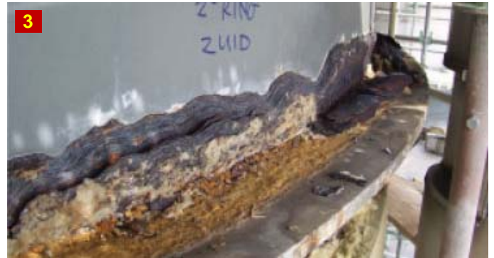
(1) and (2) – Examples of damaged insulation (3) – Corrosion resulting from damaged insulation
