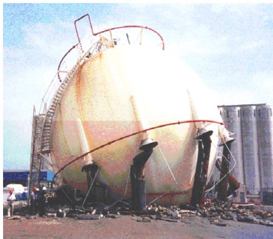
Corrosion Attacks Structural Supports
