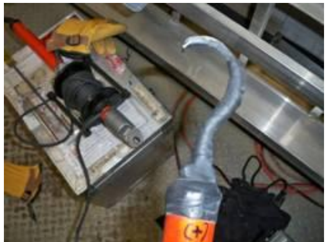
Phase Stick Hook Used to Check MCC
