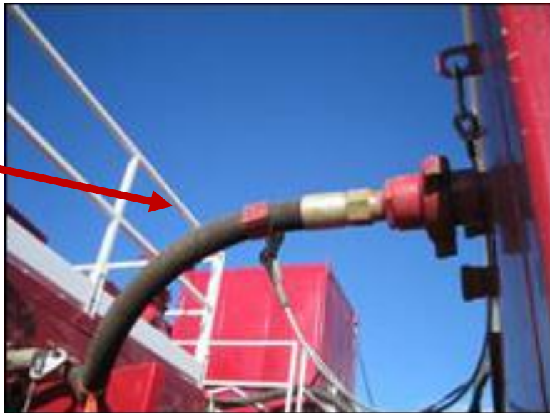
3 inch bleed off line swages down to a 2 inch hose. The 2 inch hose was replaced with a 3 inch hose to eliminate the piping restriction.
