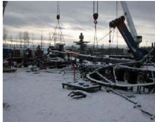
Post Incident Photograph
