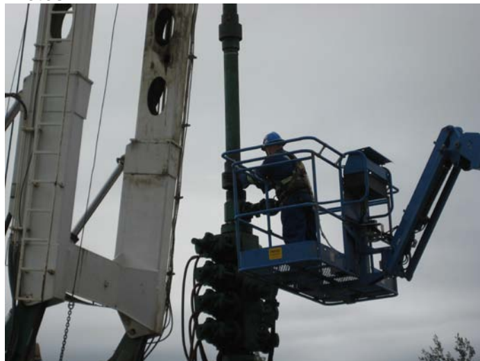
Image 1 is the position of the employee before being struck.
