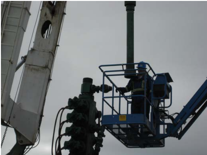
Image 3 is the employee being struck by the lubricator.
