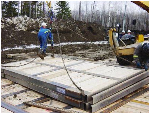
Photo #3 - Correct use of a quadruple leg sling to lift an access mat. Note: The outriggers on the lift equipment being used are not yet deployed.
