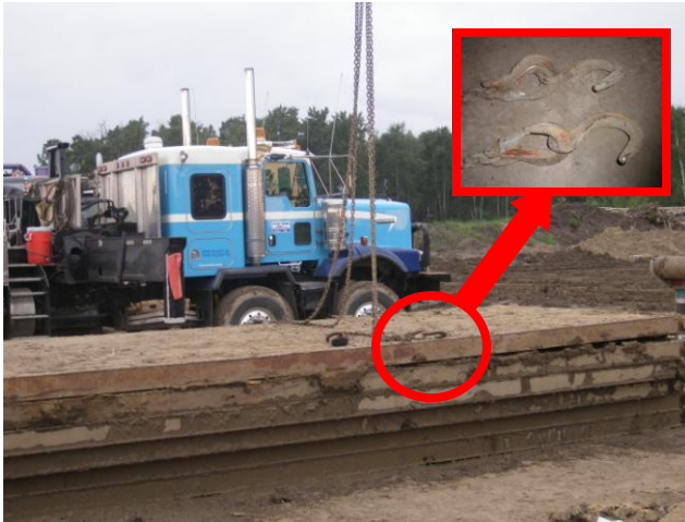
Photo #1 - Standard rig mats, no lifting shackles. Two hook system used when worker was injured. These 'pelican' hooks were removed from service.
