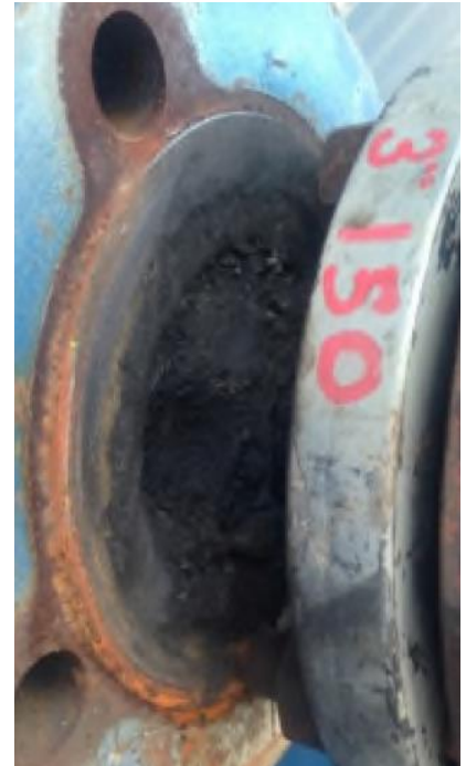
Plugged Flare Line
